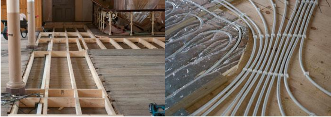
Flooring and cables for underfloor heating
